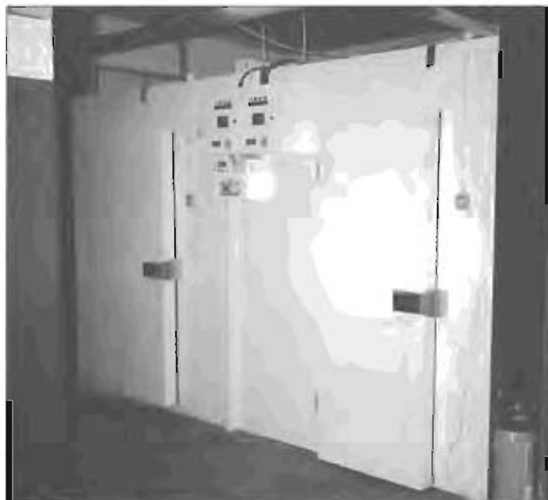
Our new fridge and freezer is installed.
